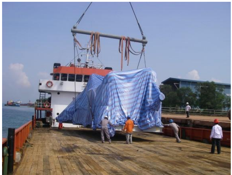
Above: Loading process. A 250-ton Kobelco crawler crane with custom-made spreader bar was used
